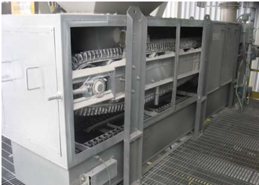
DMO Weighfeeder operating in a cement manufacturing plant.
